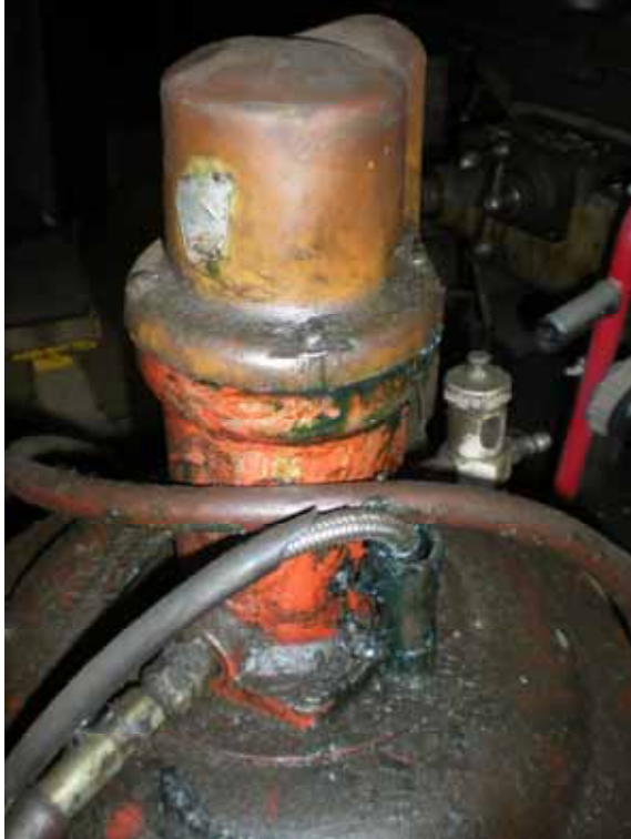
Worn Hose Leaking product No air filter
